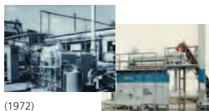
(1972) Dirt incineration system / waste fluid and waste oil incinerating system A foray into the field of pollution prevention
